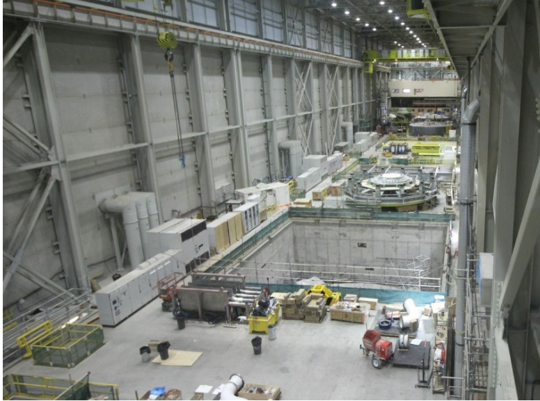
Inside the Muskrat Falls Powerhouse overlooking Unit#4
