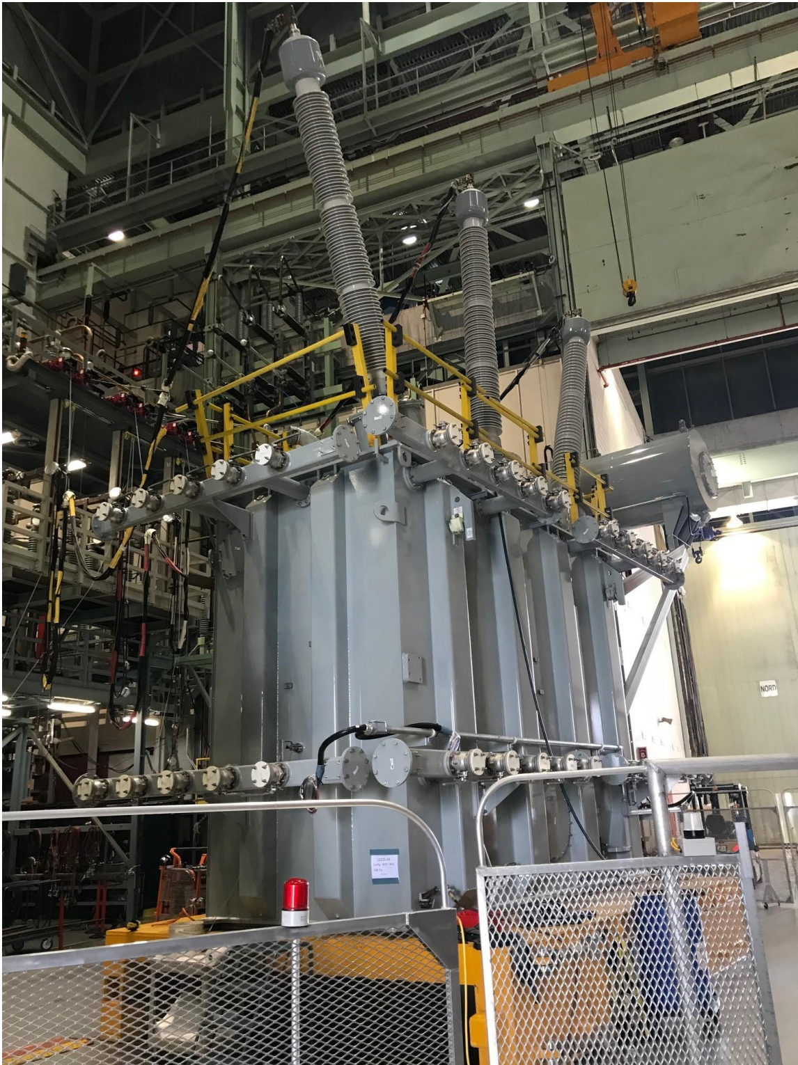
Photo 1: MFG GSU Transformer in the High Power Test Bay
