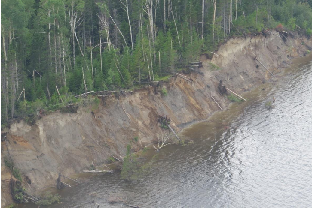
Figure 2: Active erosion South Bank, 82 Km
