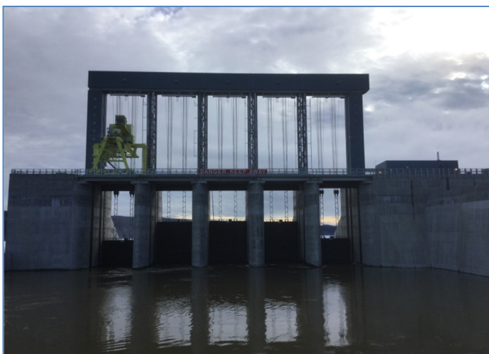
Upstream side of the spillway on May 11, 2017. Gates 1 & 5 are closed; and Gates 2, 3 & 4 are partially open. Gates are numbered 1 to 5 from right to left.
