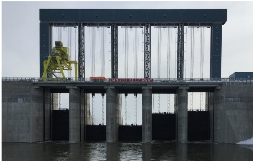
Upstream side of the spillway on March 31, 2017. Gates 3 & 4 are closed; and Gates 1, 2 & 5 are partially open. Gates are numbered 1 to 5 from right to left.
