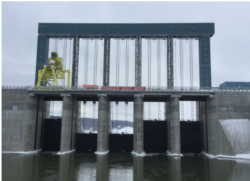
Upstream side of the spillway on March 3, 2017. Gates 3 & 4 are closed; and Gates 1, 2 & 5 are partially open. Gates are numbered 1 to 5 from right to left.
