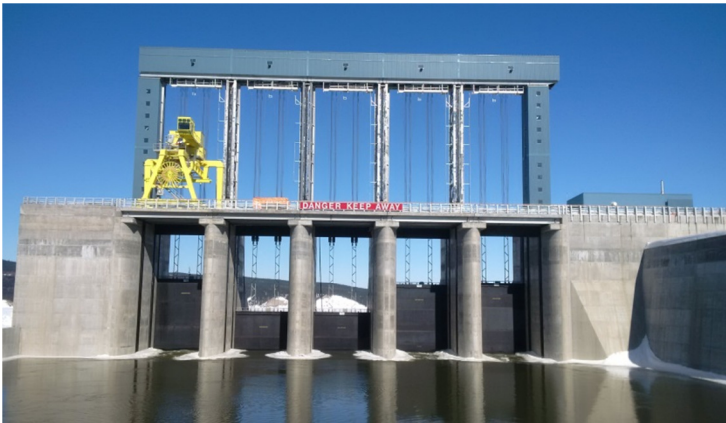
Upstream side of the spillway on March 27, 2017. Gates 3 & 4 are closed; and Gates 1, 2 & 5 are partially open. Gates are numbered 1 to 5 from right to left.
