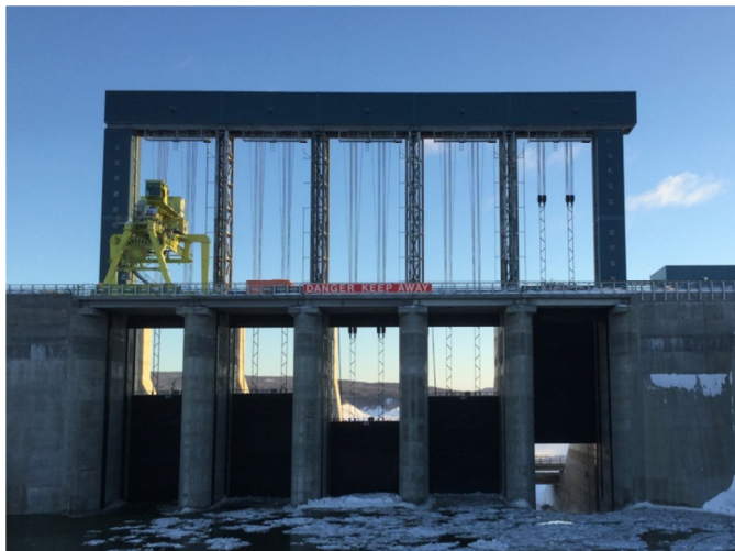
Upstream side of the spillway on February 10, 2017. Gate 3 remains closed; Gates 2, 4 and 5 remain partially closed; Gate 1 remains open. Gates are numbered 1 to 5 from right to left.
