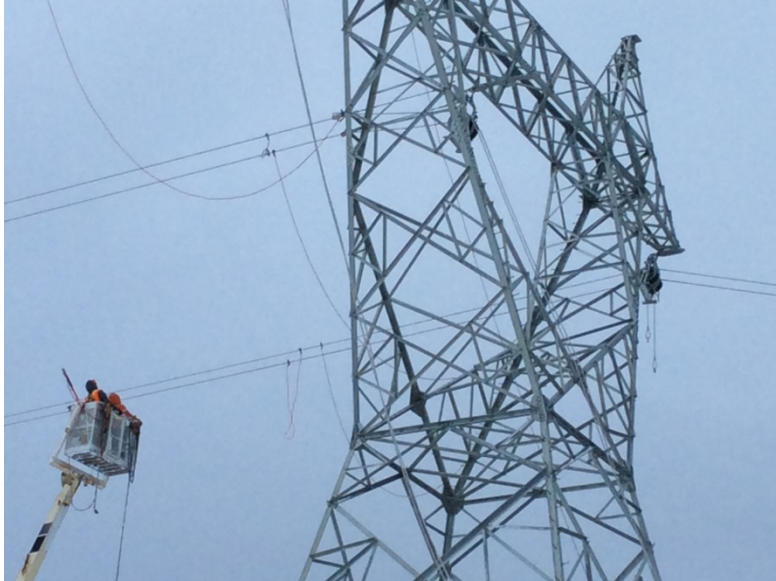
Stringing conductor wire on the transmission line from Muskrat Falls to Churchill Falls
